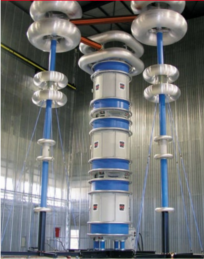
Fig. 1 HVAC resonant test system type WRM
